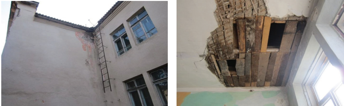
Figure 5 and 6. The deteriorating state of School #44 in Bishkek
